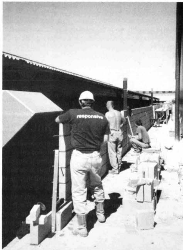
Work actively in progress: building the inner skin of the outer wall of our new "Sideways" Extension
