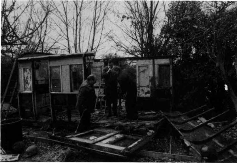
Demolition team at Kirton: the half-body of GN Suburban No. 3021 approaches the final stages of dismantling
