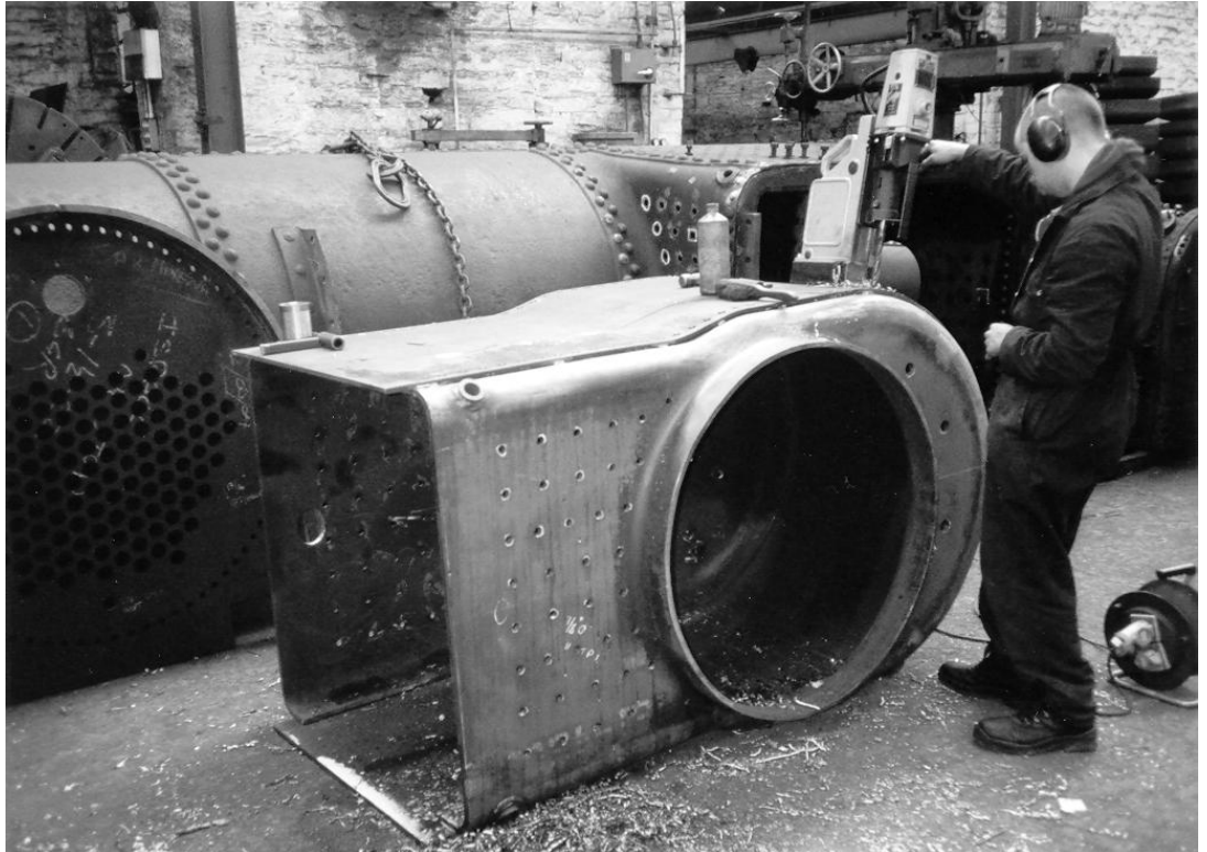
Sir Berkeley's boiler under construction at Messrs Israel Newton's, Bradford: the firebox wrapper being drilled to enable it to be riveted to the throatplate and to the backplate.
