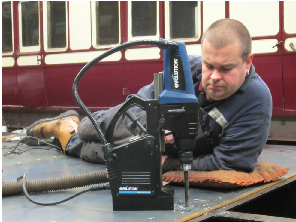
Caption Competition time? Chris Smith using our new magnetic drill as part of the process of securing the new steel sheet to the top of the underframe of the Metropolitan Railway Brake.
